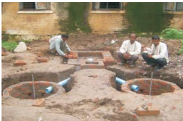
Picture 1: Construction of a Twin Pit Toilet. Both pits should be one meter apart.
